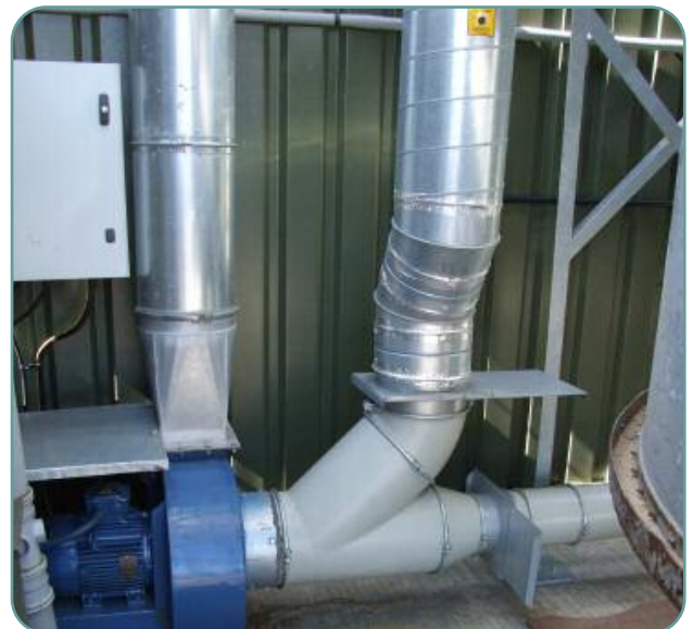
7.5kW direct coupled Paddle blade fanset, for taking milled waste from an industrial shredder and conveying into a holding silo for a waste burning & heating project.
